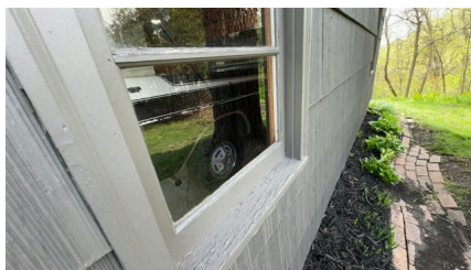
2.7 Item 4 (Picture) both garage windows
